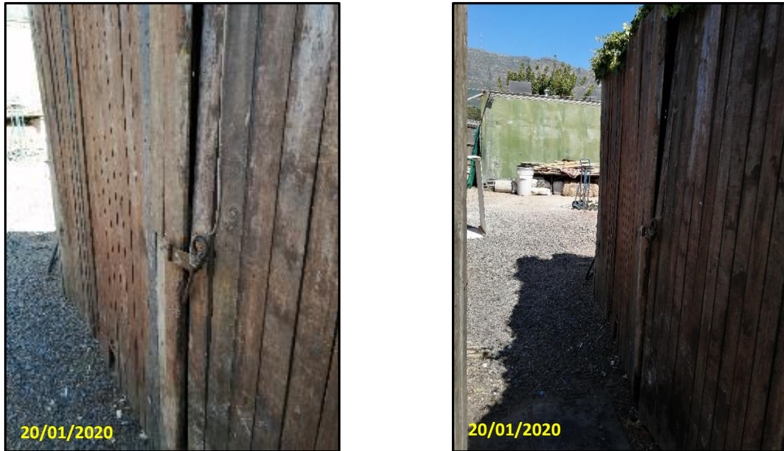
Figure 7: The bin room at The Range.
